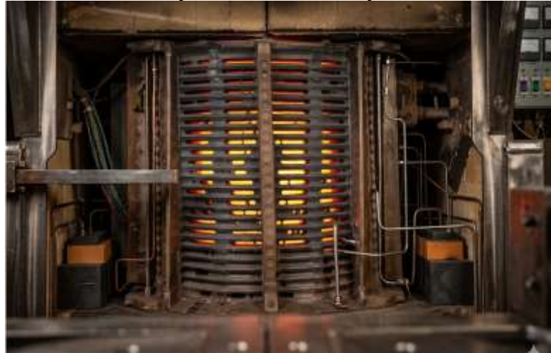
Fig. 1. Medium-frequency coreless induction furnace
